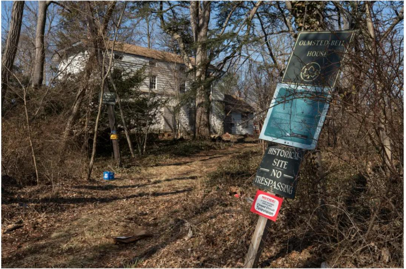
The Olmsted-Beil House in Staten Island, the one-time home of Frederick Law Olmsted, who designed Central Park with Calvert Vaux. The city bought the house about 12 years ago but it is now in disrepair. James Estrin/The New York Times
